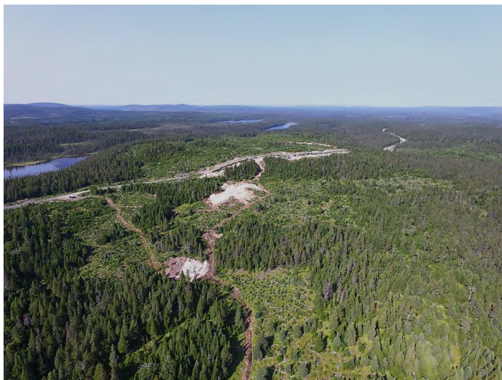
Figure 18: Sail Pond Project Area Access Road and Trenching at Heimdall Zone, looking north.
